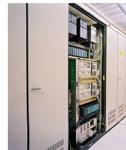
Original CJR01 Cabinet with new SPPA-R3000
