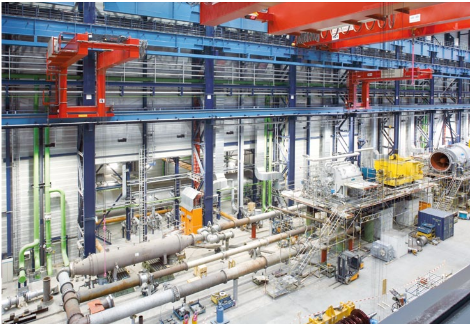
Preparation of test run
