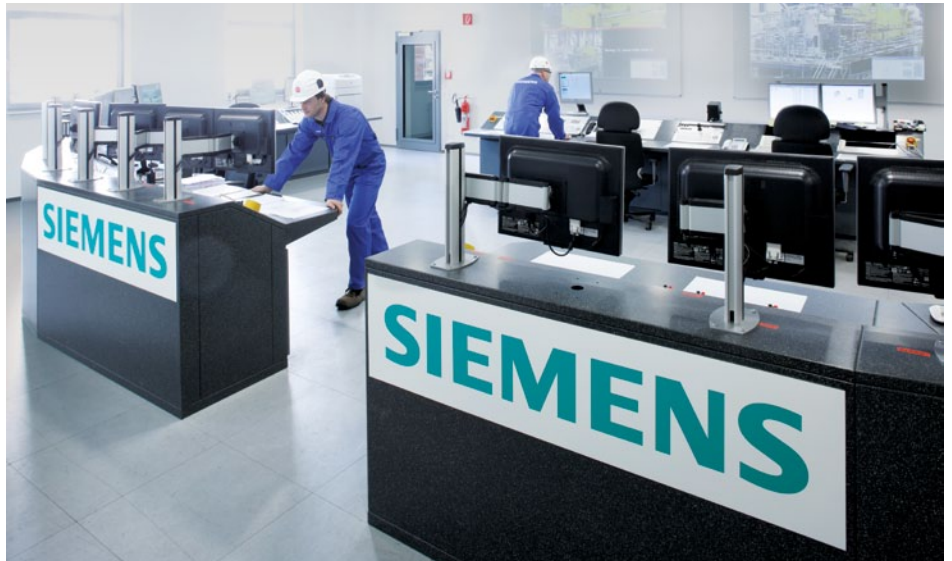
Control center in the Duisburg Mega Test Center
