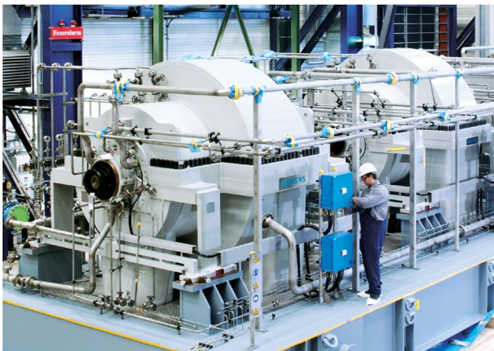
Compressor train for petrochemicals
