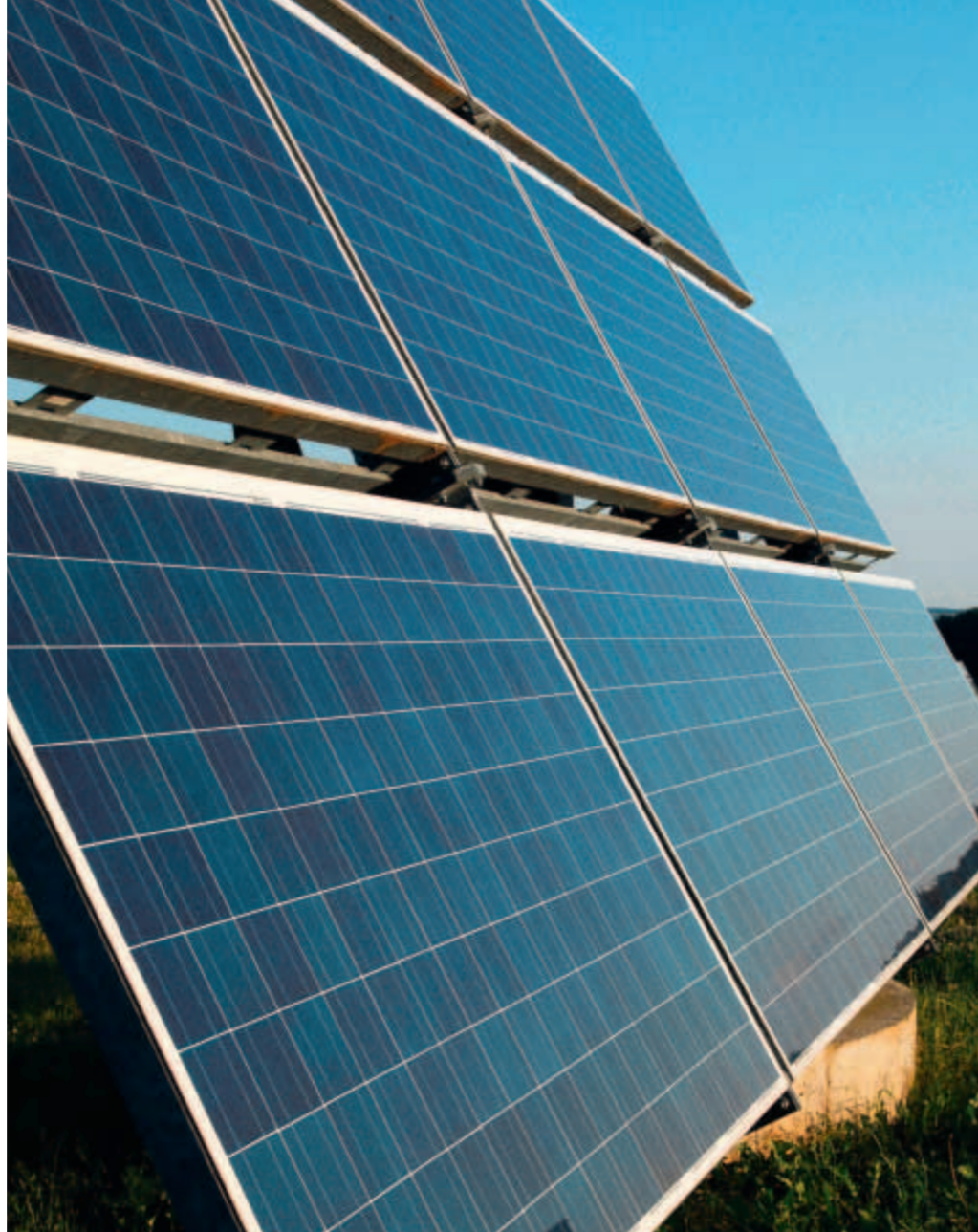
Using prefabricated, lightweight aluminum supports like these, Siemens built a photovoltaic plant in Italy in just one month that serves 350 families.
