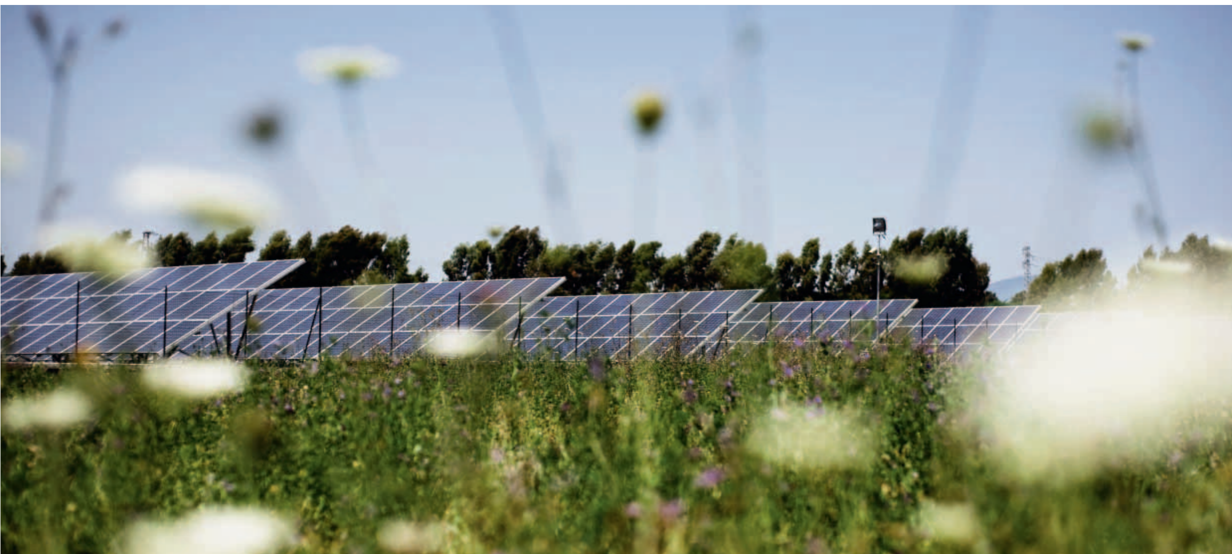
Impressions from Ferrarelle PV power plant, Italy.
