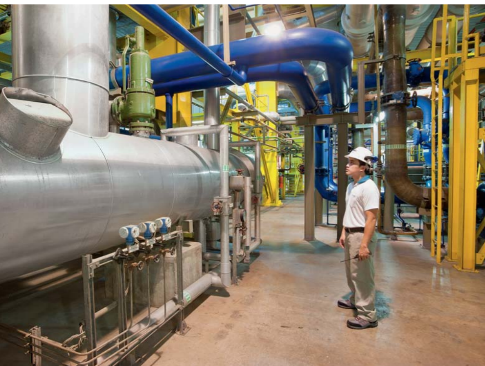
Efficient O&M services ensure low emissions at the Santa Rita power plant near Batangas City.
