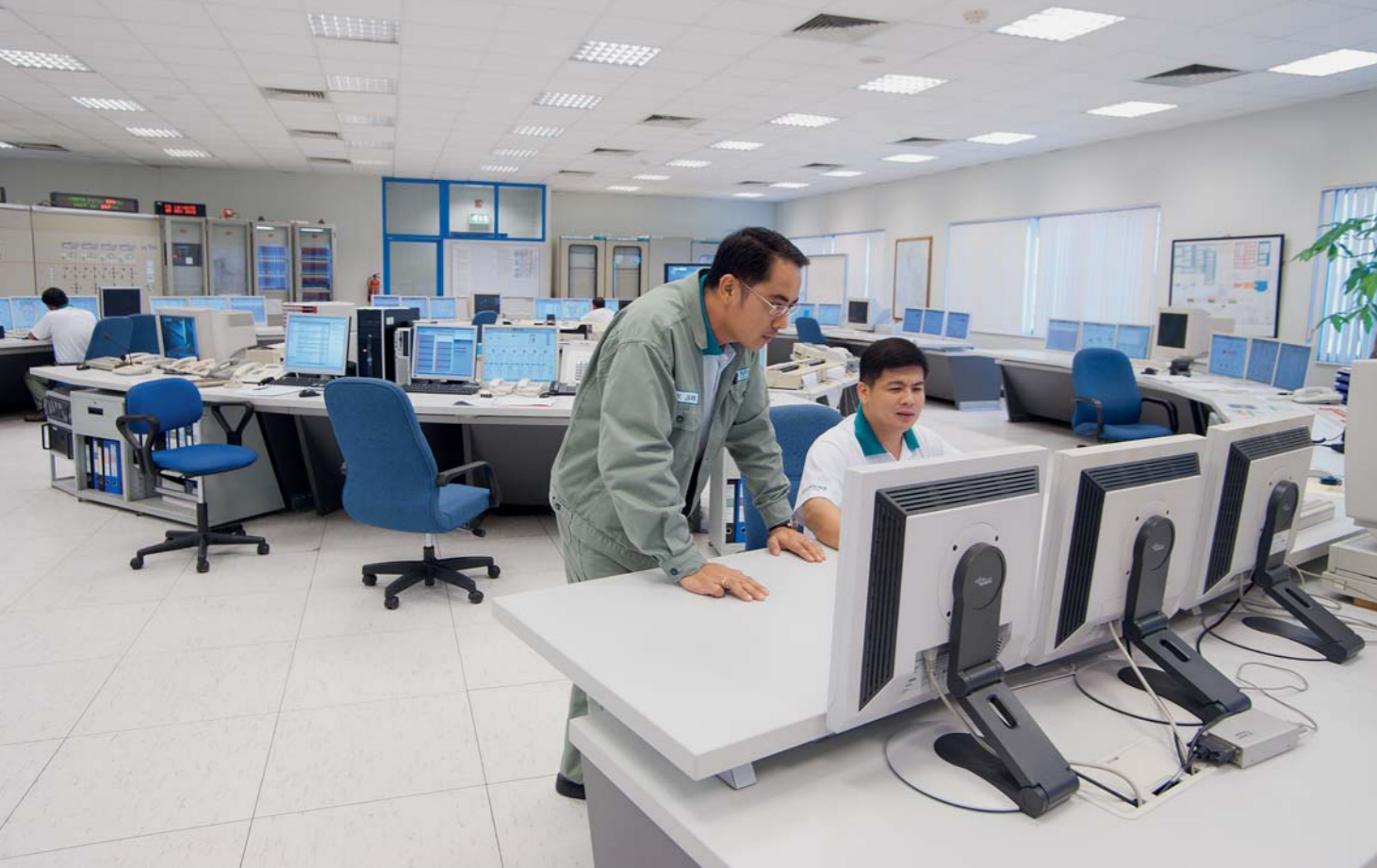
Siemens handles plant administration on a day-to-day basis. The heart of the installation is the control room.
