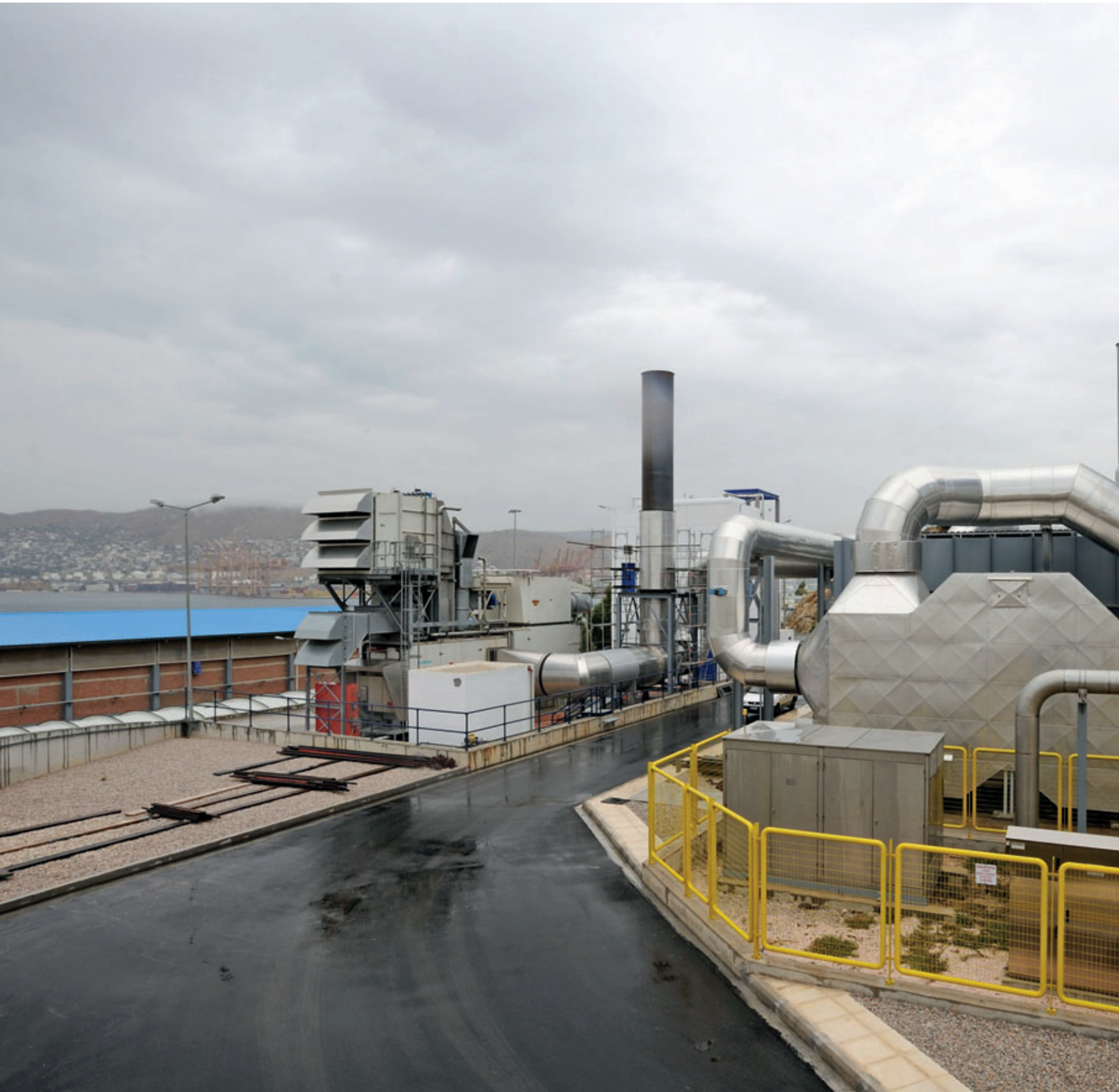
The new SGT-400 cogeneration package (left) on Psyttallia Island off Athens. The heat of the gas turbine exhausts is used for sludge drying in the facility to the right.
