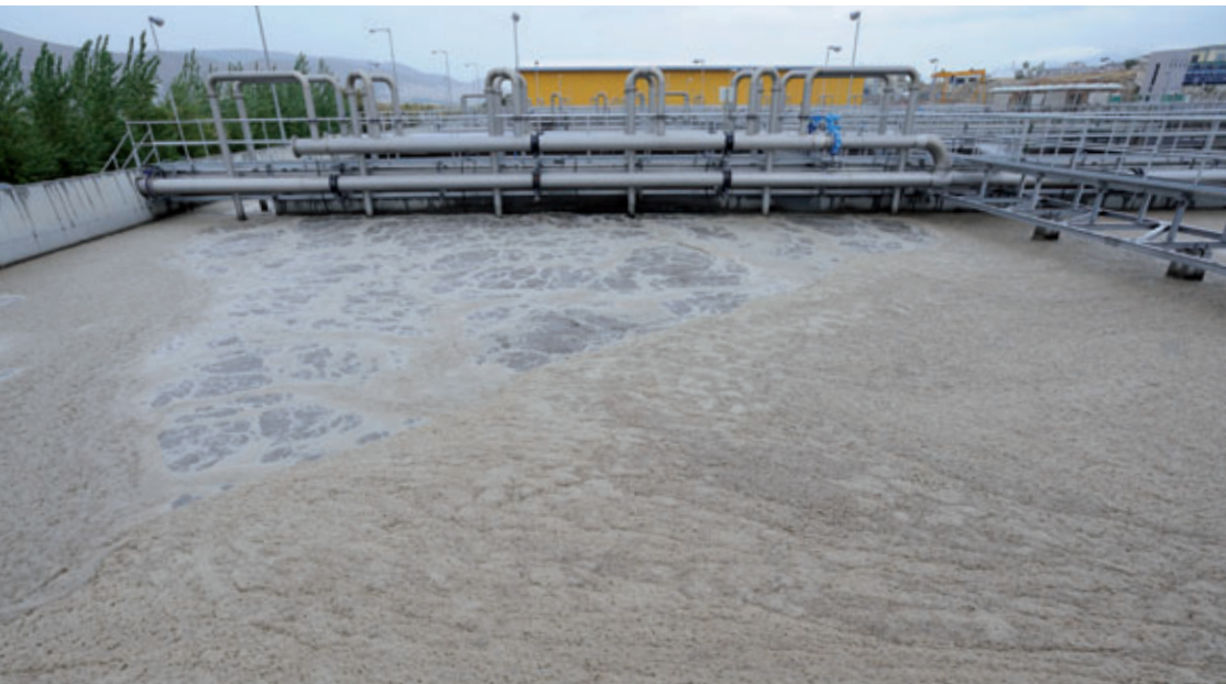
Energy consumption accounts for some 95 percent of the operational costs of aeration units.
