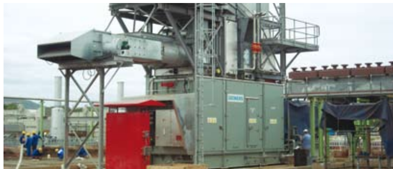
Two SGT-400 pipeline compressor sets for Sasol Technology (Pty) Ltd, installed at the Komatipoort compressor station in South Africa.
