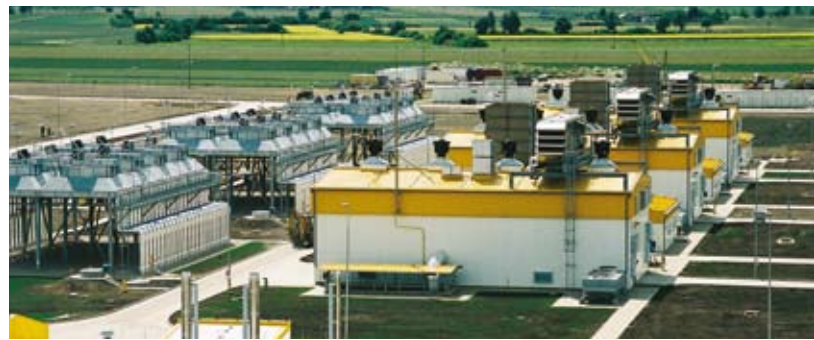
Four units were installed at a pipeline compressor station in Kondratki, Poland.
