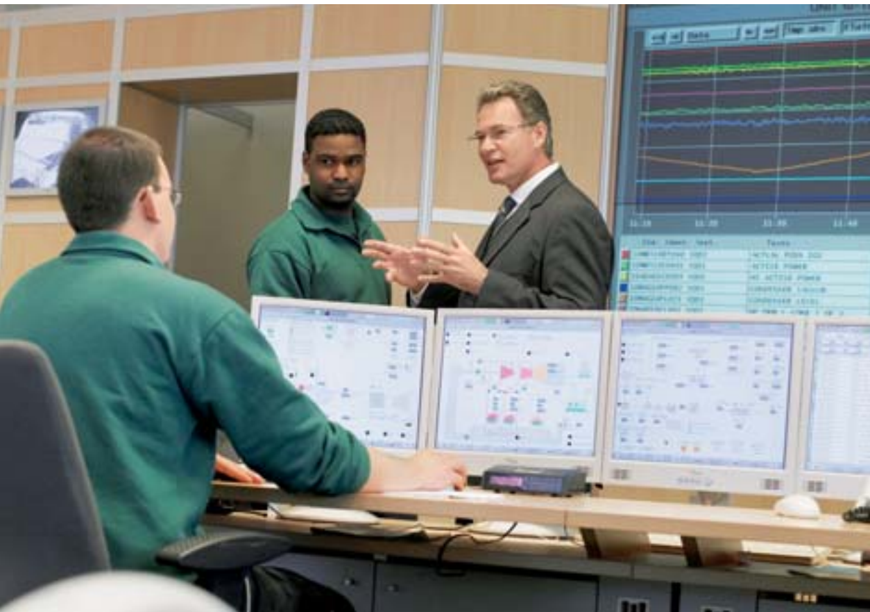
SPPA-T3000 Control System
