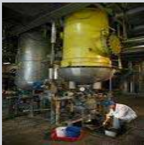
Siemens Fuel Gasifier
