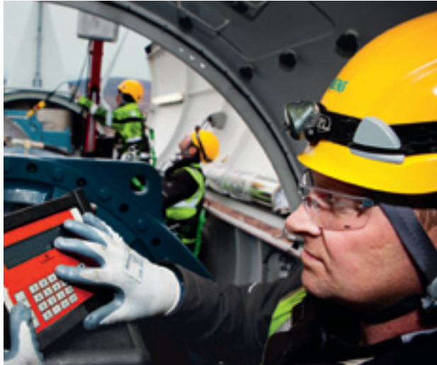
Service technician inside nacelle
