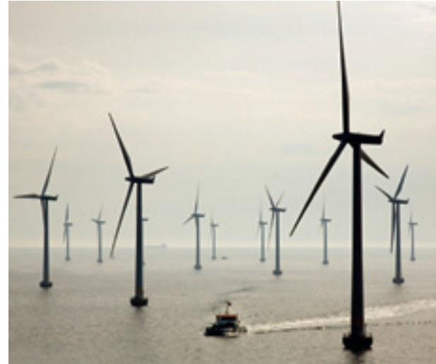
Lillgrund offshore wind farm, Sweden
