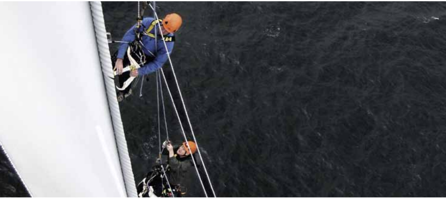
Specially trained Siemens Service Rope Access Technicians install a power curve upgrade package
