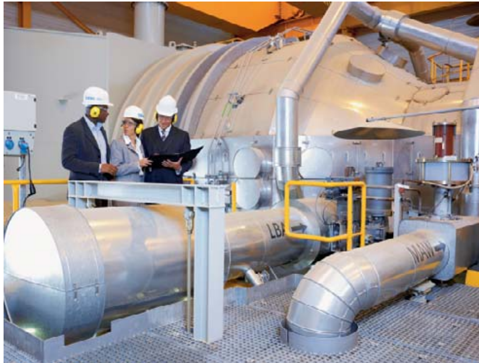
SST5-3000 steam turbine in the combined cycle power plant (CCPP) Ribatejo, Portugal
