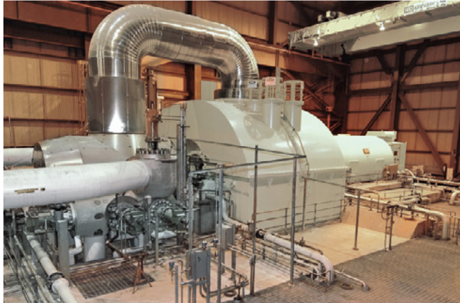
SST6-5000 steam turbine in the combined cycle power plant (CCPP) Osprey.
