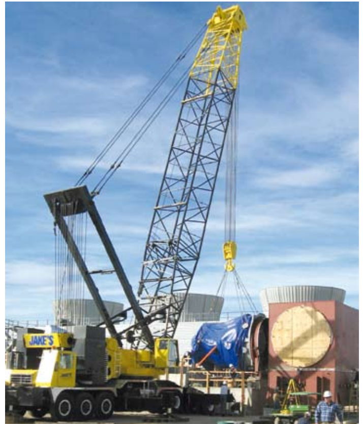
Installing the SST-700 LP turbine on the concentrated solar power plant in Boulder City, Nevada, USA.
