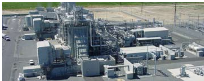
In the Walnut Energy Center CCPP in Turlock, California, a 100 MW SST-900 dual-casing steam turbine in reheat configuration uses the heat from two gas turbines.
