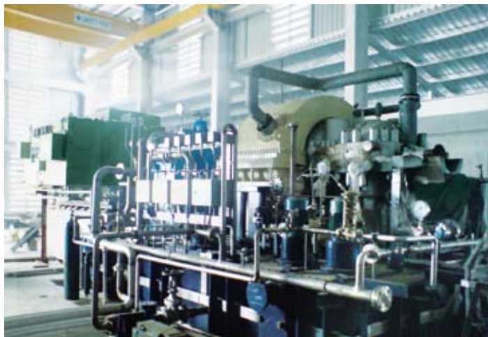
Bangkok, Thailand: A 9.9 MW steam turbine generator set in a power plant of the Power Prospect Company Ltd.
