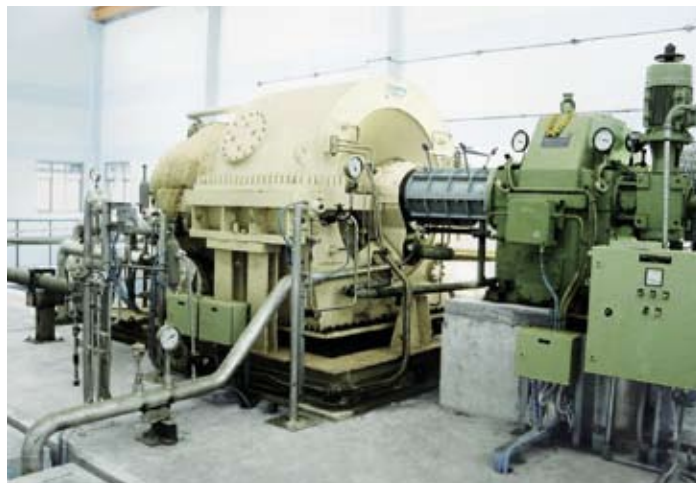
Roi Et, Thailand: 9.9 MW turboset for the Bua Sommai Electricity biomass power plant.
