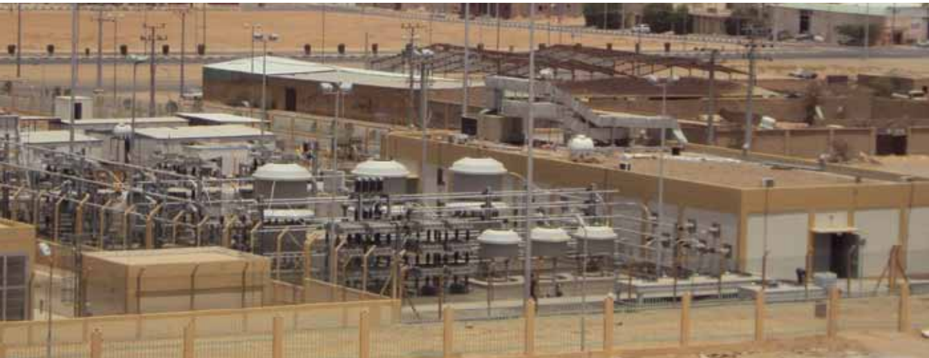
Fig. 8.1: Turnkey SVC Project
