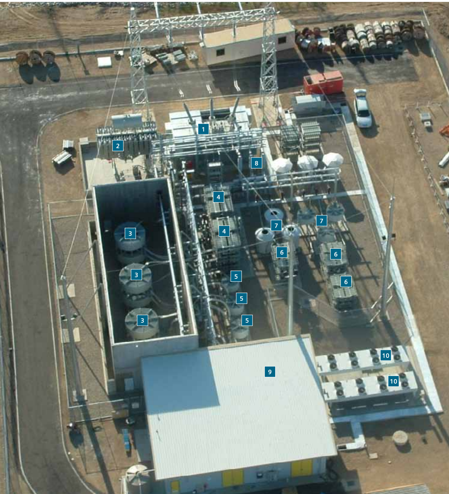
Fig. 4.17: Strathmore SVC, Australia (1 TCR/1TSC/3 Filter)
