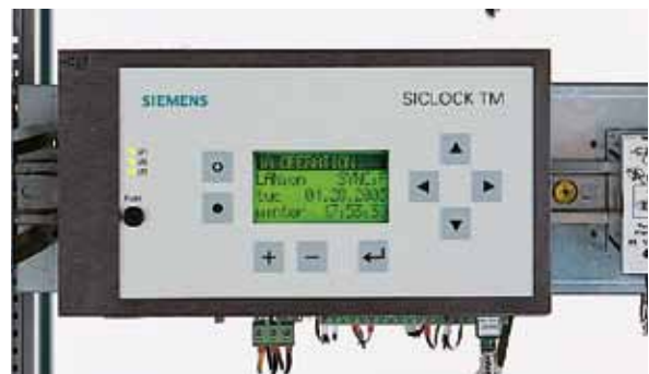
Figure 4-9: Time Synchronisation System
