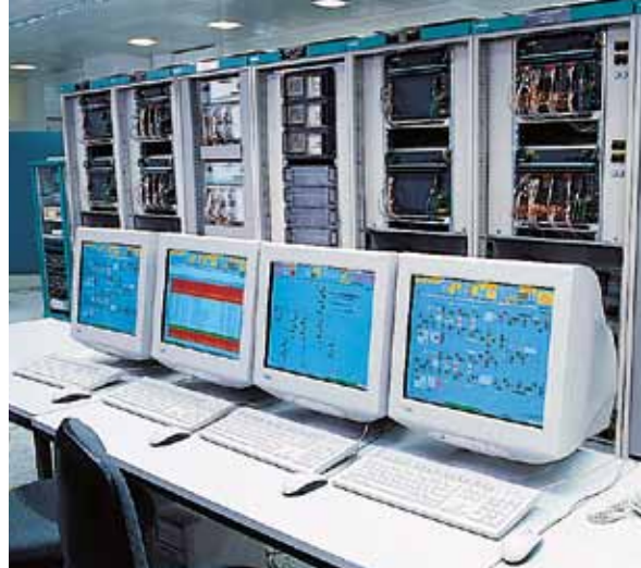
Figure 4-2: HMI System at the Functional Performance Test
