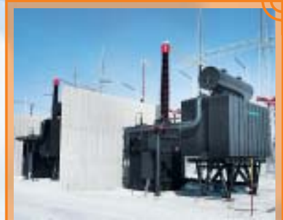
Up to very high voltages: 110-MVar single-phase shunt reactor, 735 / \sqrt{3} kV for Canada.
