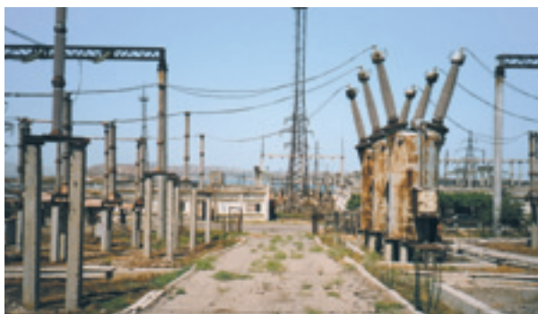
HV substation before modernization
