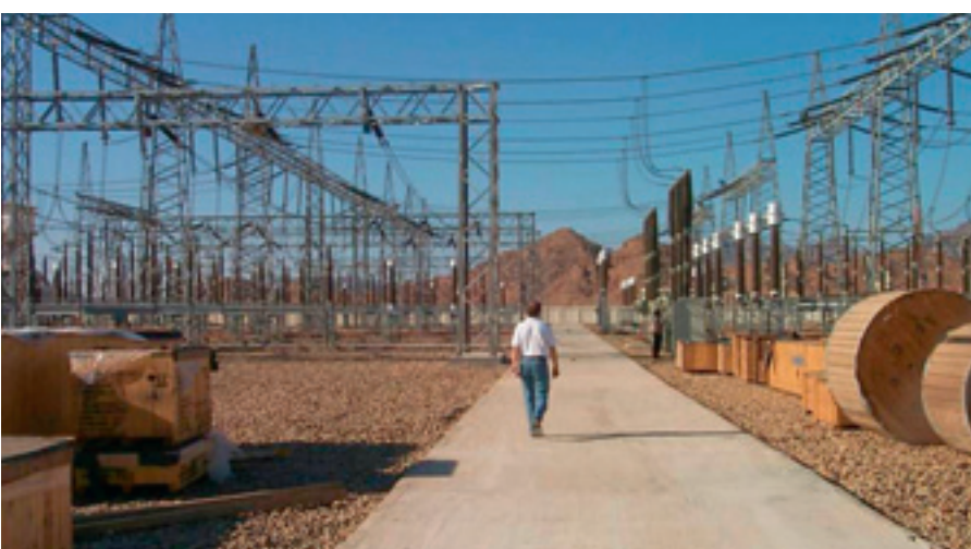
220 kV, Sharm-el-Sheikh, Egypt
