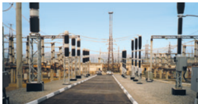
HV substation after modernization
