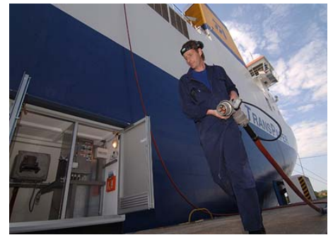
Figure 3: Siharbor solution for power supply from the shore
