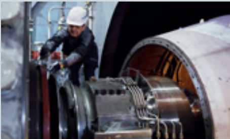
The quality standards demanded for power-plant service are implemented through a comprehensive maintenance concept.
