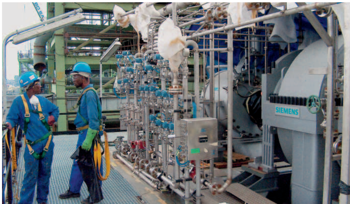
At Sasol's coal-to-liquid plant in Secunda, South Africa, a series of chemical processes convert coal into synthetic fuels.
