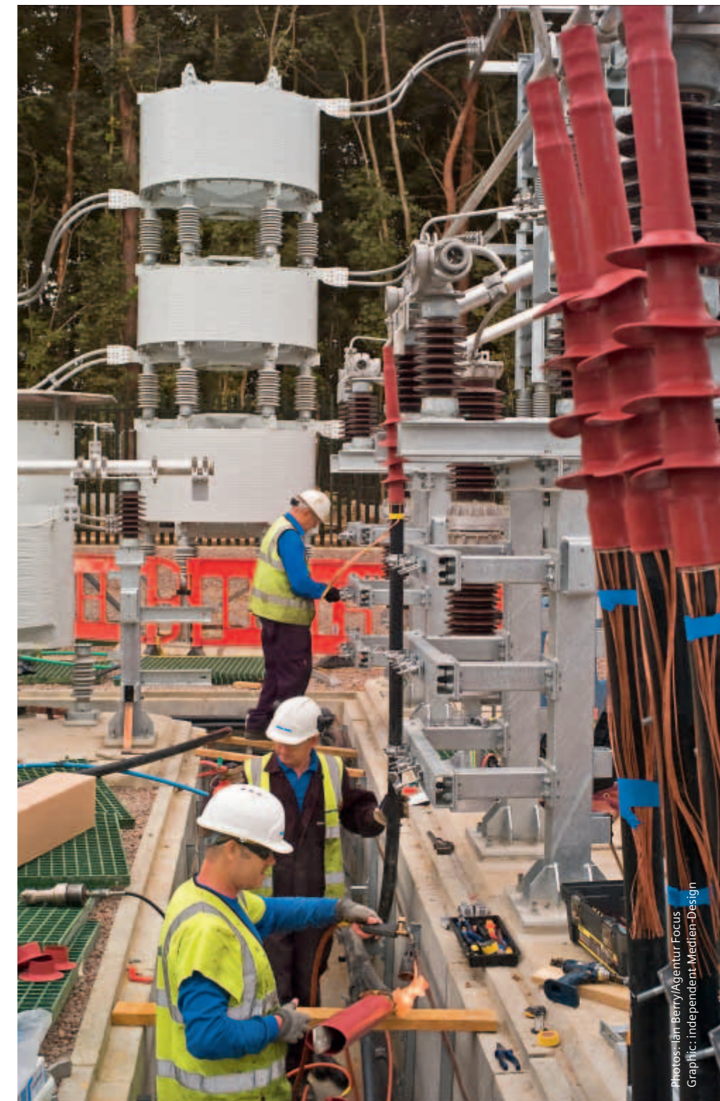
Greater Gabbard onshore substation at Leiston: power quality for grid access of world's largest wind farm – components for three SVC Plus systems "under construction."
