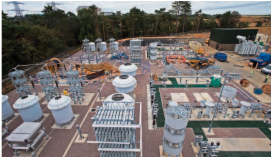
Construction site at Leiston with two of three compensation circuits. The substation connects the 132-kV AC sea cables from the offshore platform with the grid on the mainland.
