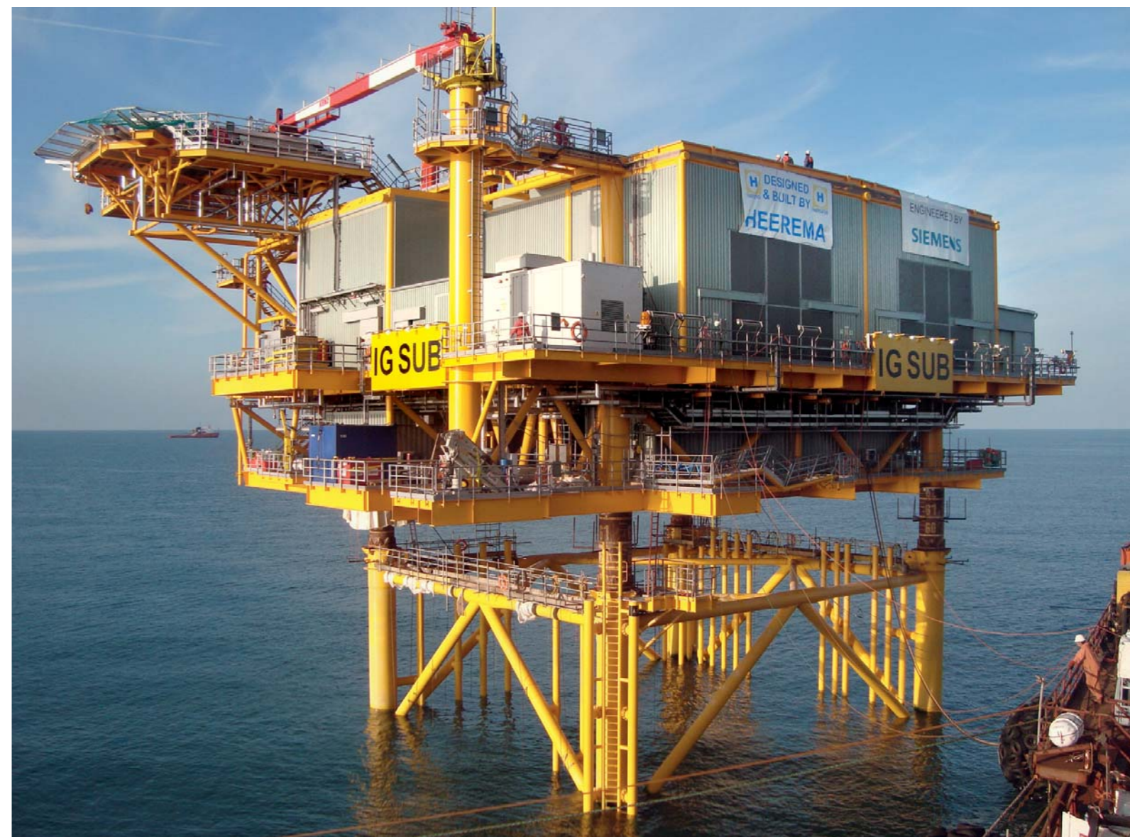
At the 500-MW Greater Gabbard site off the coast of Suffolk, 140 Siemens wind turbines of 3.6 MW each will produce carbon-free electricity.
