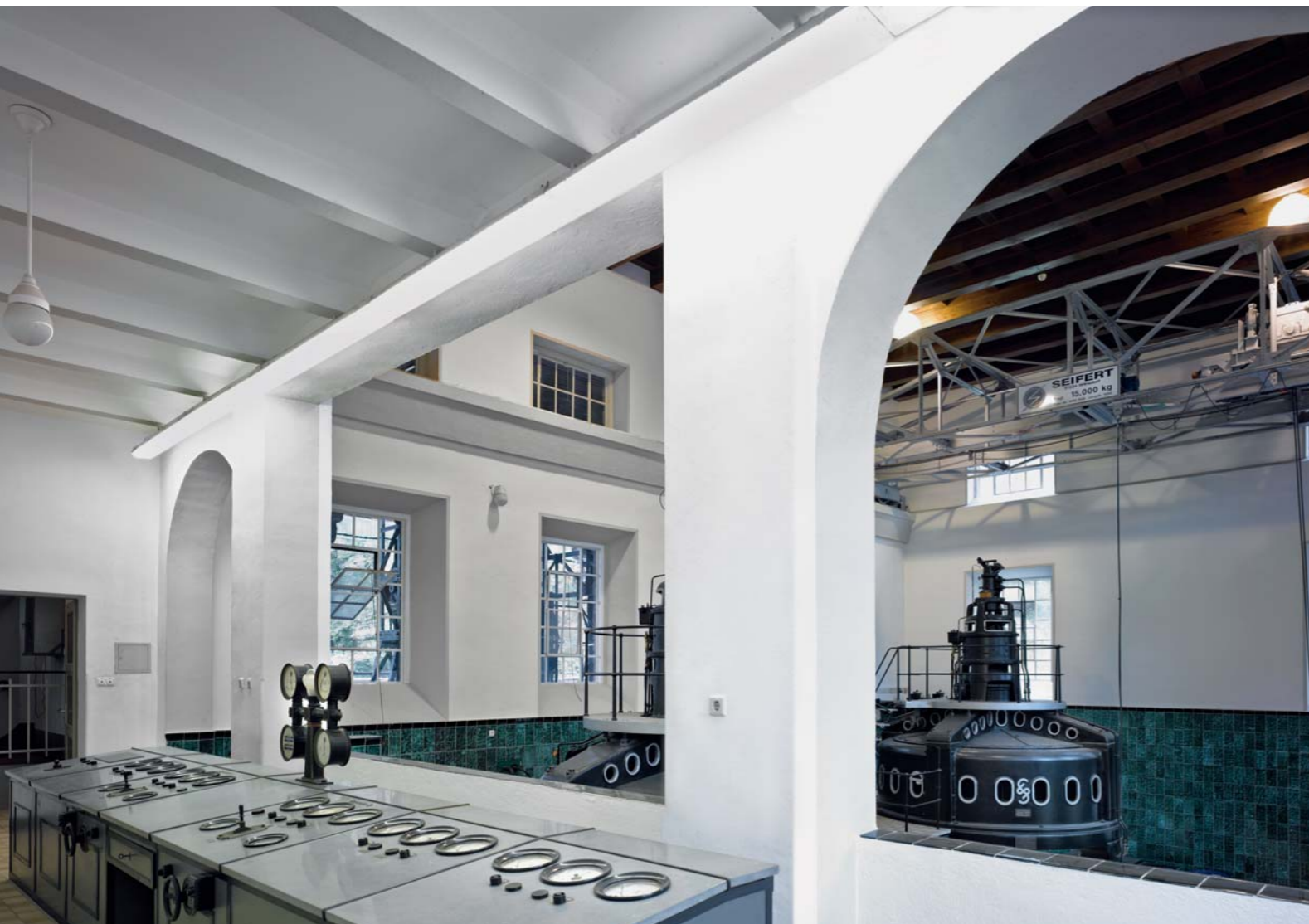
The vintage marble control desk faces a pair of Siemens-Schuckert three-phase synchronous alternators.
