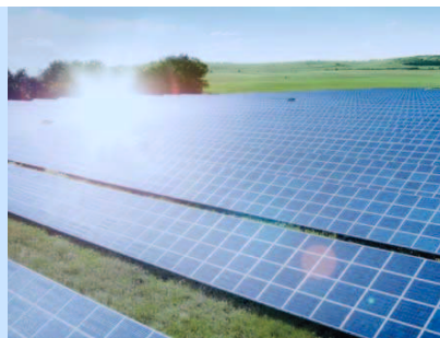
Photovoltaic panels from Siemens will capture solar energy to provide environmentally friendly power to thousands of homes in east central Italy.
