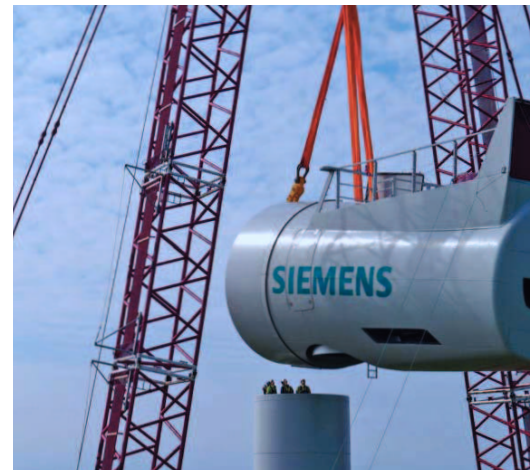
The nacelle of the SWT-6.0-120 prototype being hoisted to the top of the tower.
