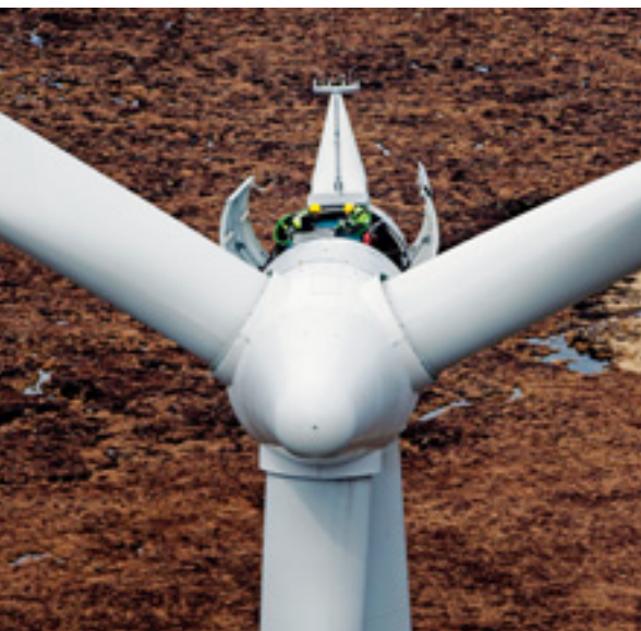
Service crew at work on a SWT-2.3 nacelle at Farr wind farm, Scotland
