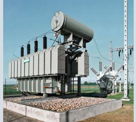
Transmission transformer for the Bürgerwindpark Lübke-Koog
