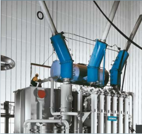
15 generator transformers Three Gorges, the world's largest hydroelectric power plant
