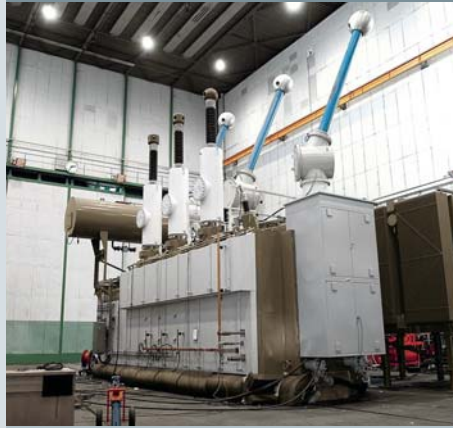
Four autotransformers with extremely low noise for a US power supply company
