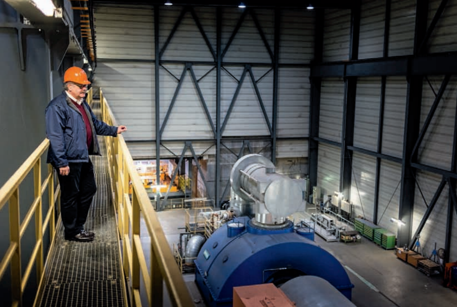
Thomas Zimmerer, KMW's Technical Service I&C Engineer, takes pride in the innovative heating concept.
