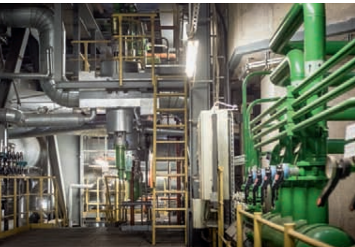
The steam reuse concept allows the KMW plant to stay in hot-start mode for a longer time.
