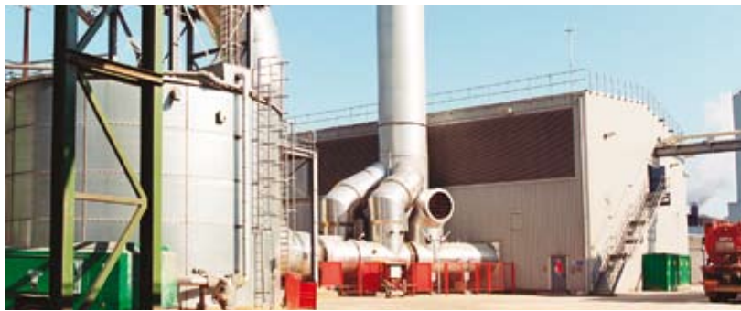
Two SGT-300 gas turbines provide Norbord with electricity and heat at their board manufacturing plant in Scotland, UK.
