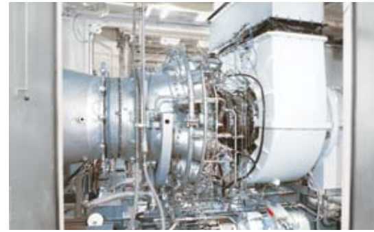
SGT-300 core engine test facility.
