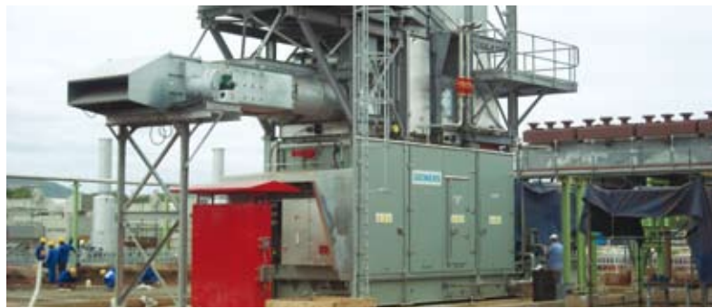
Two SGT-400 pipeline compressor sets for Sasol Technology (Pty) Ltd, installed at the Komatipoort compressor station in South Africa.
