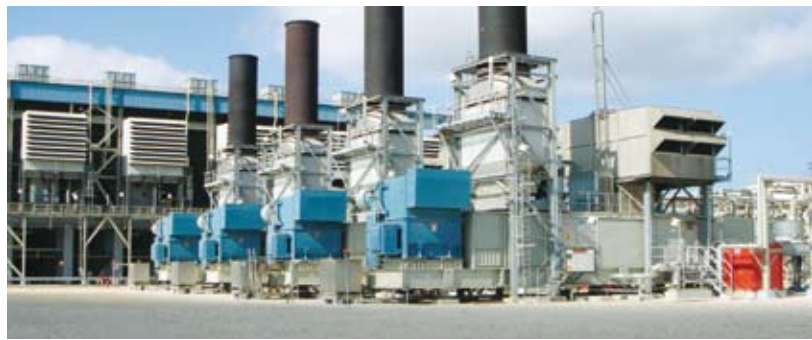
Four SGT-500 units installed in Egypt to power an LNG plant.
