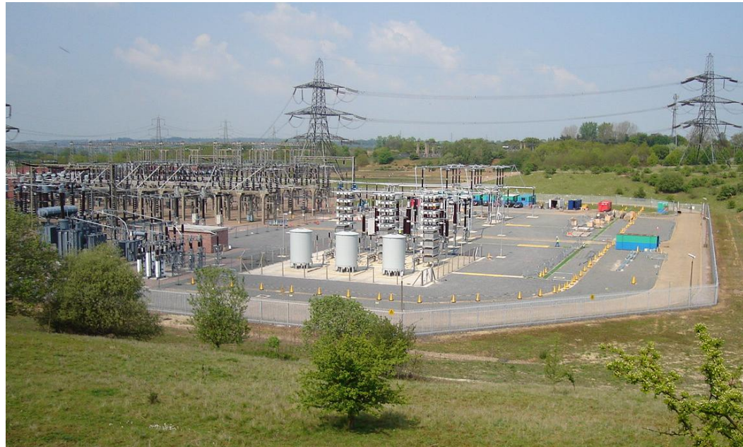
The picture shows a MSCDN for National Grid Company, U.K.
