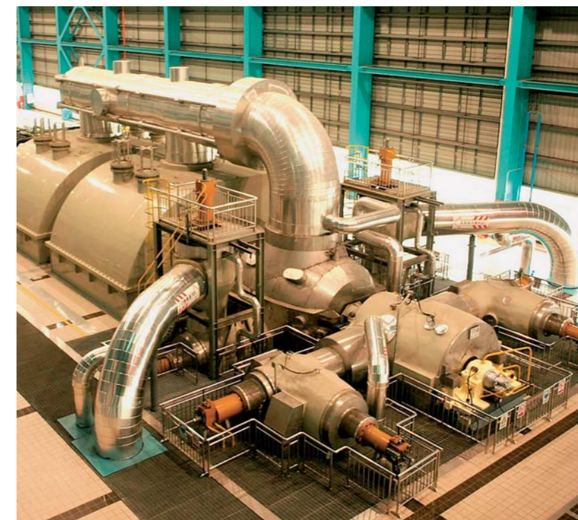
The Waigaoqiao III Power Plant: a great benchmark for utilizing coal in a more efficient and cleaner way.
